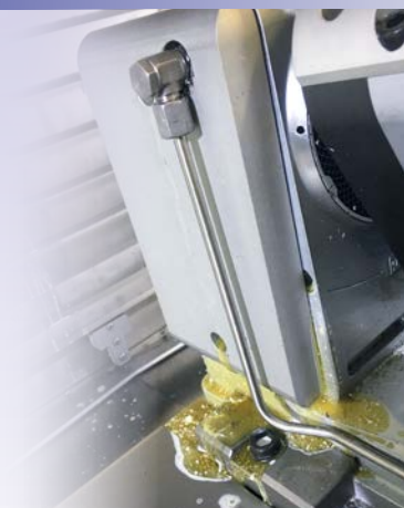
severe oil loss
